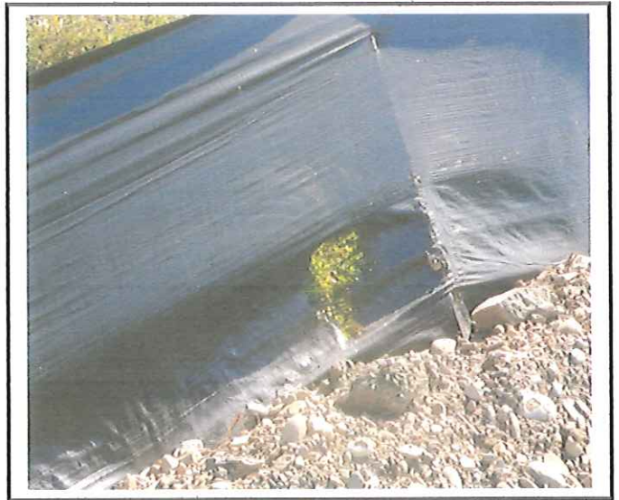
Holes in silt fence around entire site that require repair.
