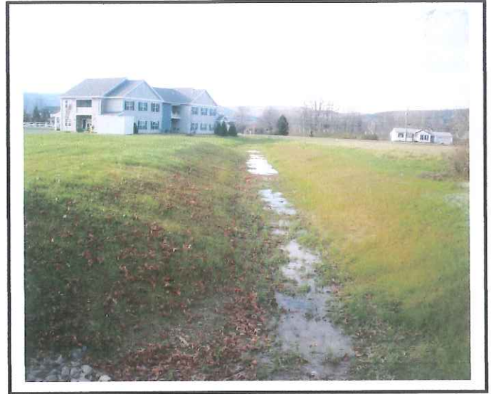
Vegetated open swale BCD has standing water.
