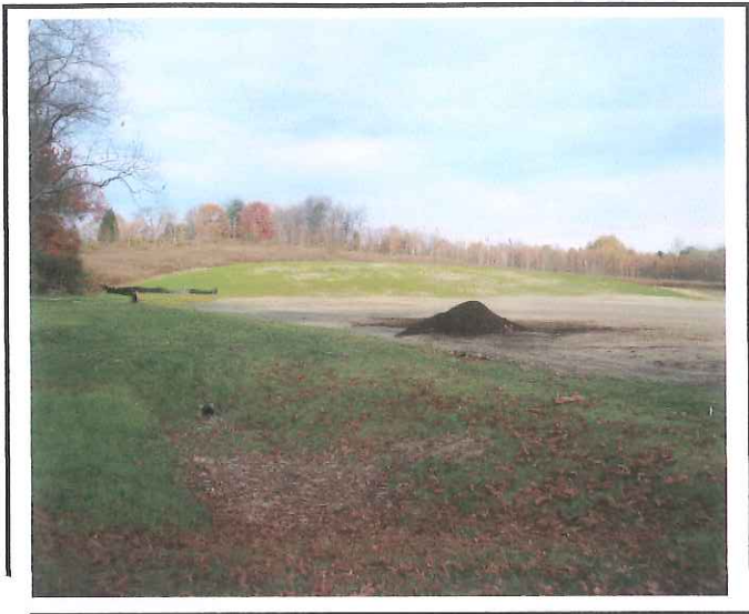
Contractor Yard has some bark mulch stored there. The fill area has been stabilized.
