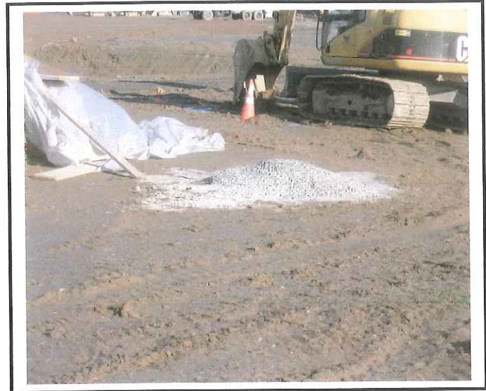
Concrete washout was full so someone washed out next to it.
