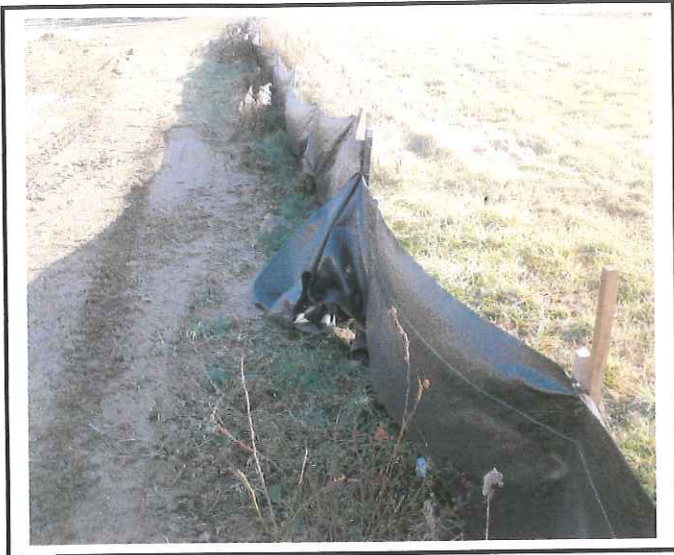
Silt fence needing repair.
