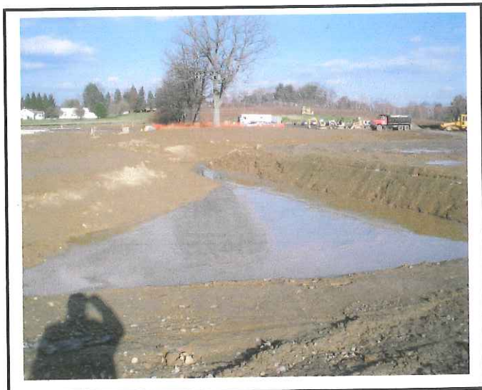
Infiltration K will need stabilization.
