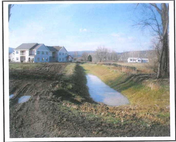
Infiltration trench BCD- Flat area was stabilized in November. But then it was utilized for building panel storage. Needs stabilization now that panels are up.
