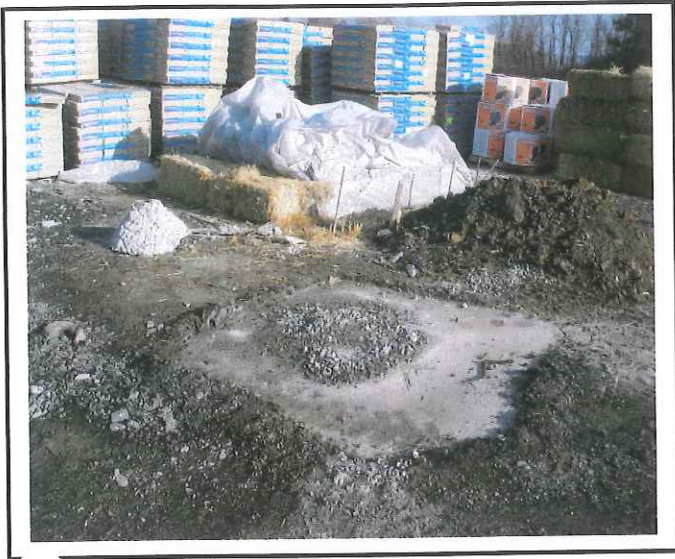
Concrete wash out in contractor yard was moved. A truck washed out next to the area that the washout was located.
