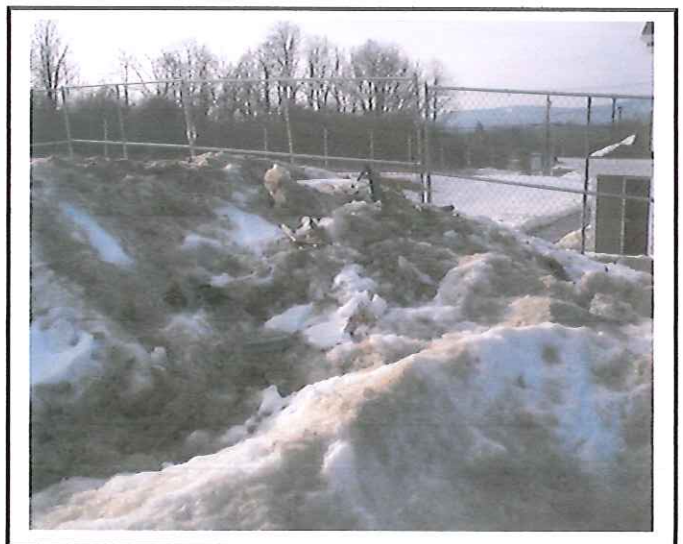
Catch basin buried under snow.
