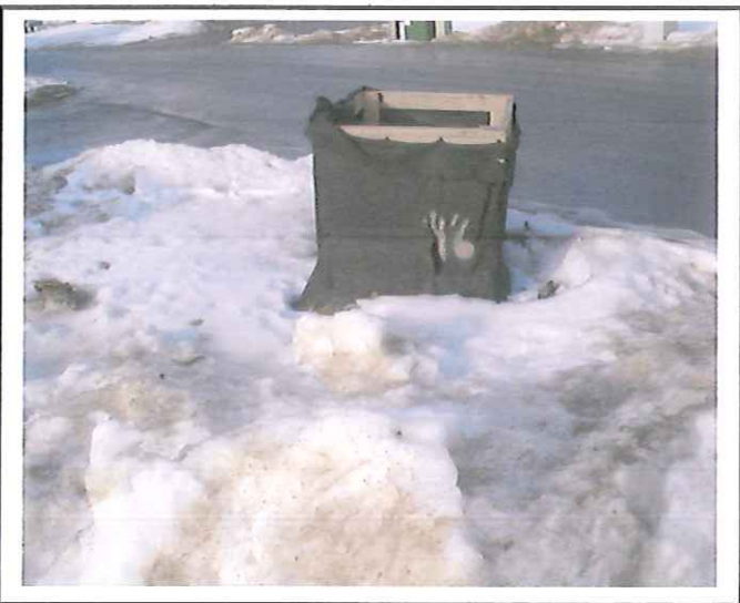
Stapled patch on drop inlet protection does not meet standard. Replace all fabric.
