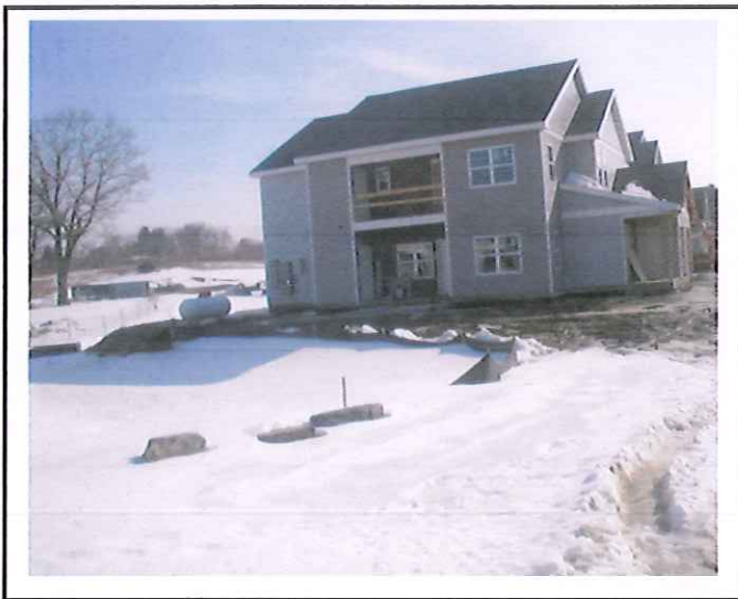
Silt fence requires maintenance.
