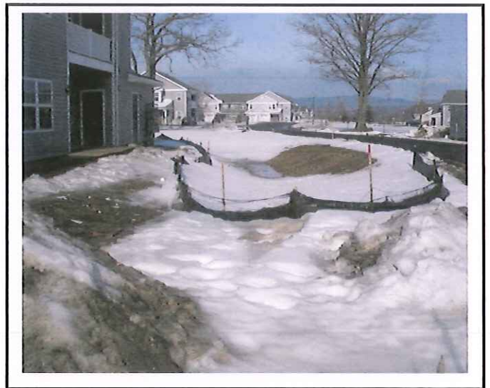
Silt fence requires maintenance.
