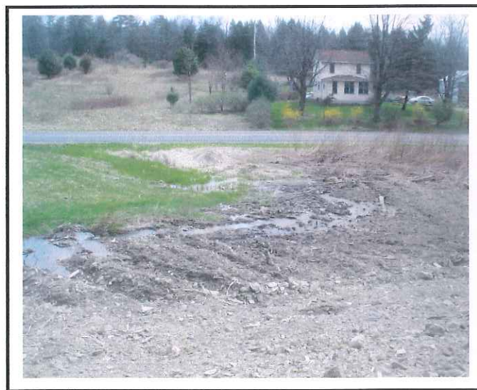
No separation between construction and outlet of existing pond.
