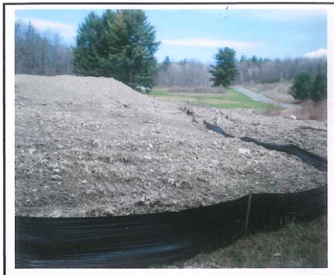
Area of disturbance. No bare soil has been stabilized.
