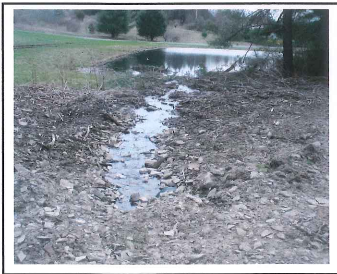
Drainage from hillside has not been re-directed but put through a culvert pipe.
