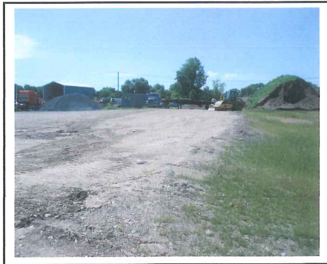
Looks like new fill material from separate facility has been added and drainage flows directly into pond.
