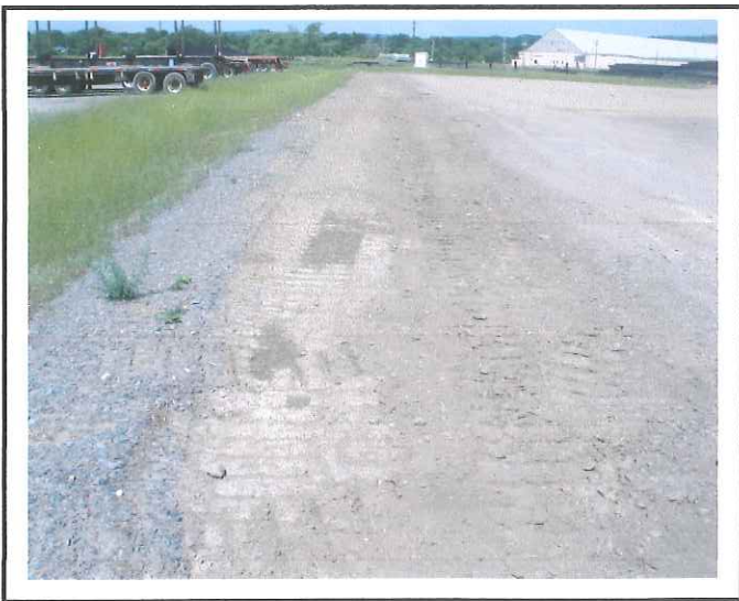
Rain Garden without mulch-6" depth is not achieved.
