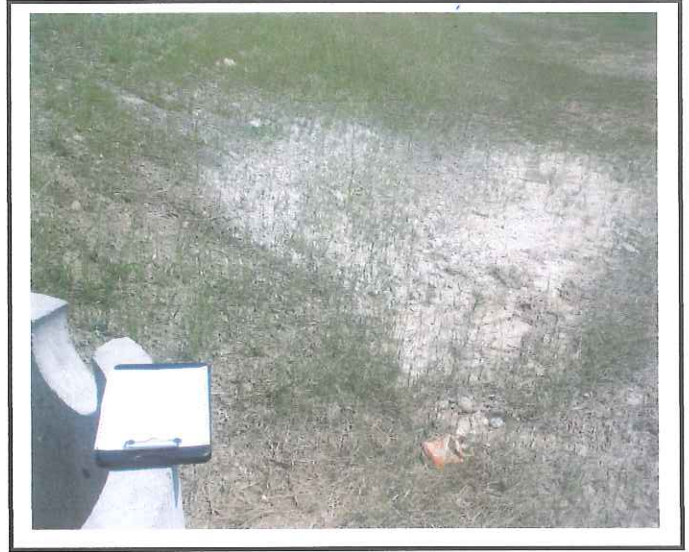
Concrete was washed out onto the side slope of the stormwater pond.
