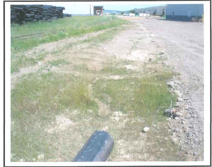
Swale is undefined and there is no rain garden installed.
