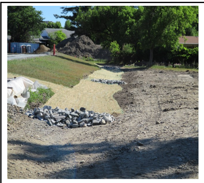
Drainage swale is not constructed according to drawing.
