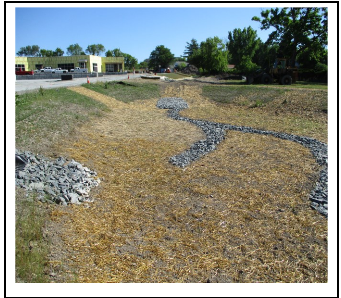
Stormwater retention basin at south end of property requires seed and more mulch.
