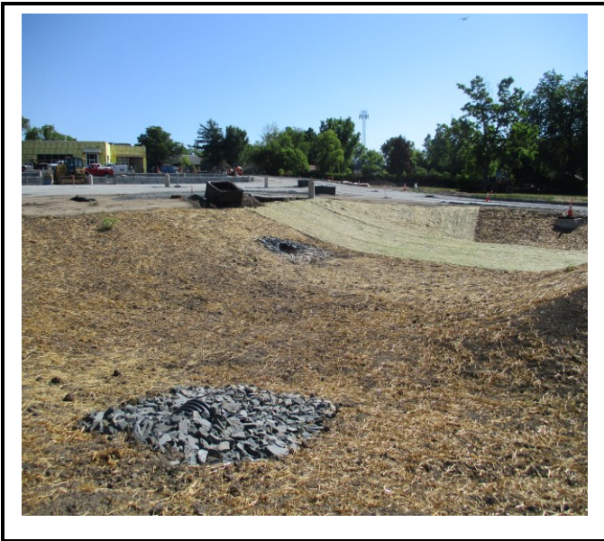
South end stormwater basin. Area has not been seeded and mulch does not cover soil as needed.
