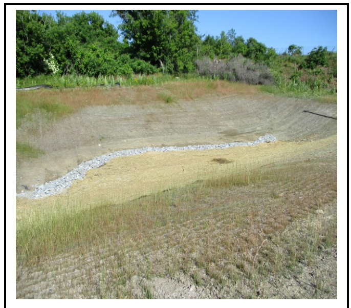
North end stormwater basin. Grass is not growing well.
