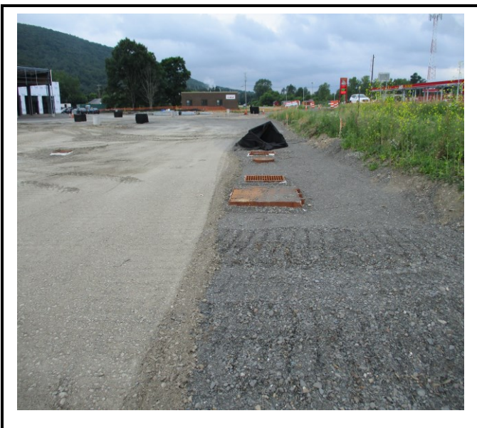
Catch basin and water quality unit that are direct tributary to underground infiltration system are open and unprotected from runoff.
