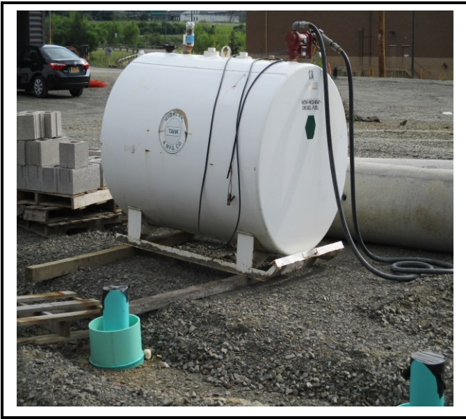
Diesel tank has been moved directly next to open observation ports of the underground infiltration system. Pollution prevention issue.
