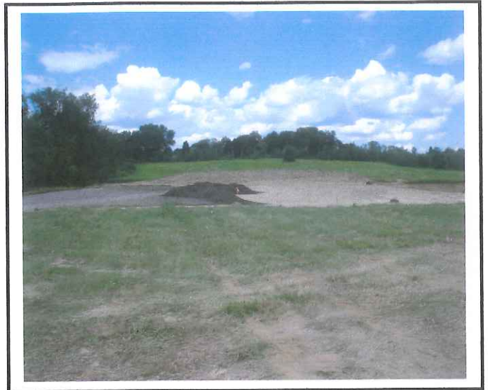
Contractor yard and soil stockpile. Contractor will be stabilizing the face of the stockpile.
