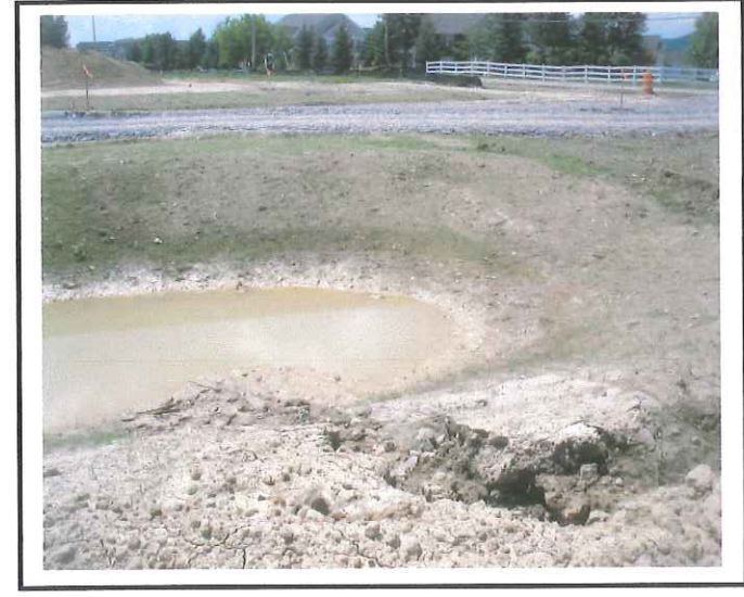
Infiltration trench A- major erosion has started on the side slope.
