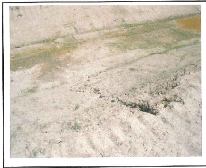
Erosion started on the side slope of infiltration BCD.
