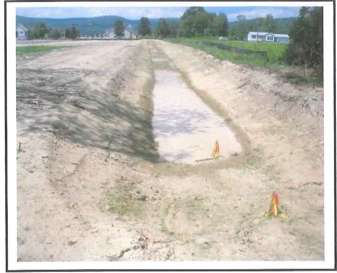
Infiltration trench BCD is still holding water.
