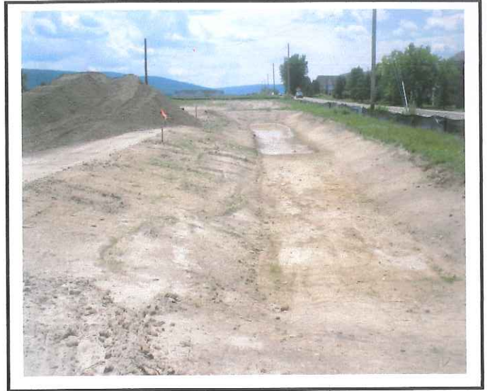
Infiltration trench F2. Soil stockpile is too close to the edge of the basin (spoke with Dave of Wenzel).
