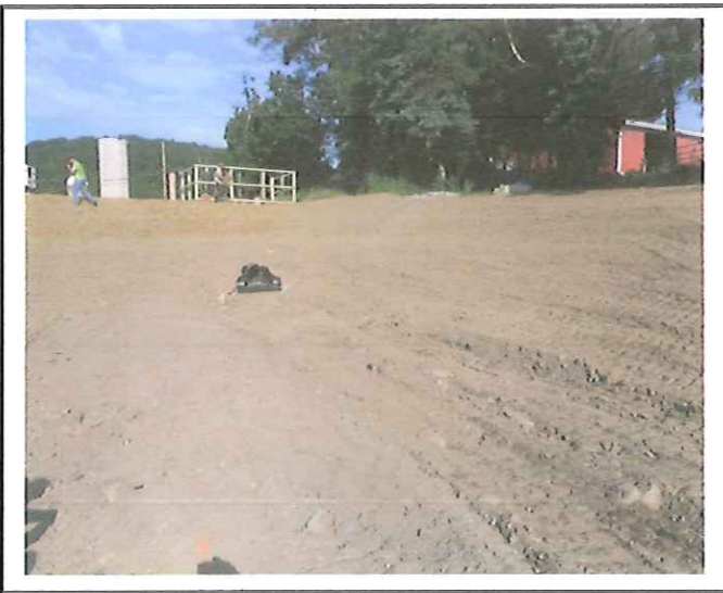
Pipe discharging into forebay- outlet protection, rock lined swale and clay liner not installed.
