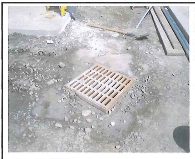
It looks like something has been washed into the yard stormwater drainage grate-this drain should be protected.
