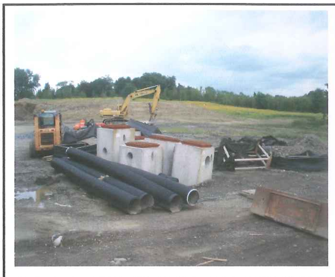
Contractor yard is getting cleaned up. The soil stockpile is being graded for final stabilization.
