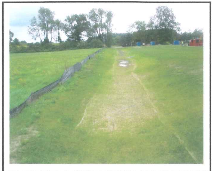
VOS BCD has been re-shaped and graded. It now looks to be 2 feet deep and no water left the site in the last storm.
