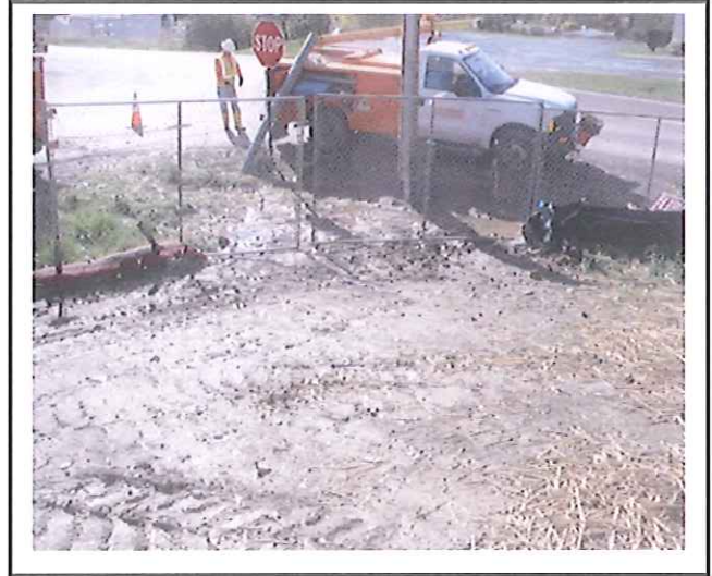
Silt fence, that NYSEG replaced, needs to be replaced.
