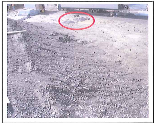
Erosion is occurring on side slopes and check dams are not functioning.
