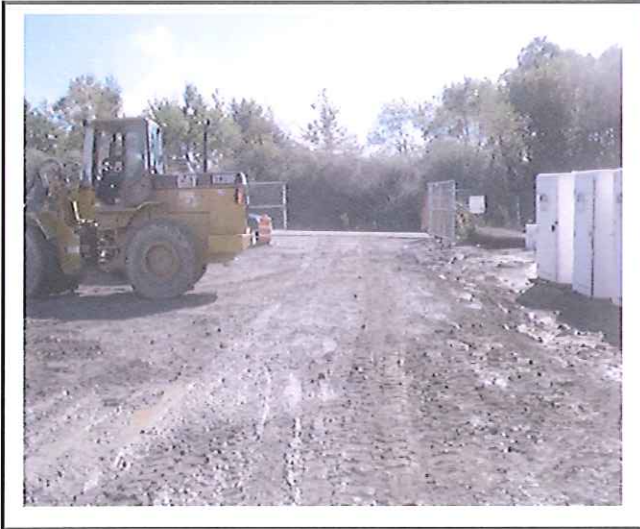
Construction Entrances- Both require maintenance and Gardner Road needs to be cleaned up.
