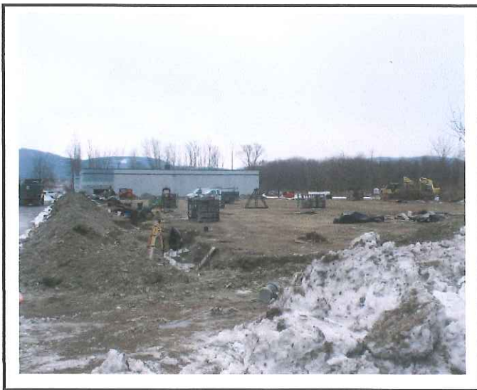
Areas disturbed are only the areas where the footer is being formed and poured.
