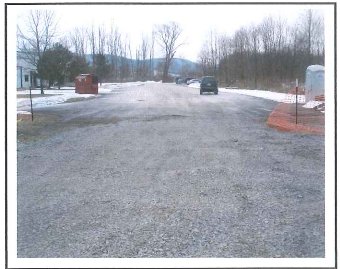
Minimal tracking off construction entrance. Continue to monitor for tracking off site.
