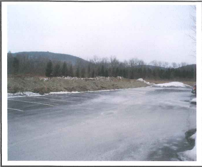
Soil stockpile next to parking area is missing the silt fence that the SWPPP and Qualified Inspector call for.
