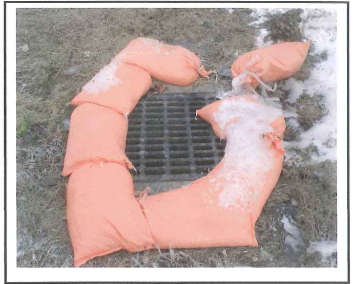
Drop Inlet protection- this is not the approved one but they would not be able to get that on installed this time of year. We will continue to monitor.
