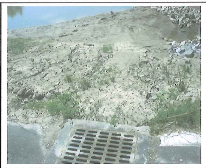
Erosion occurring on the side slope of the pond from water bypassing the catch basin.
