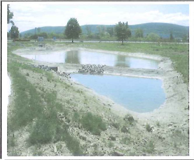
Pond water has dropped from the lack of rain. You can see the locations of the forebays and weirs.
