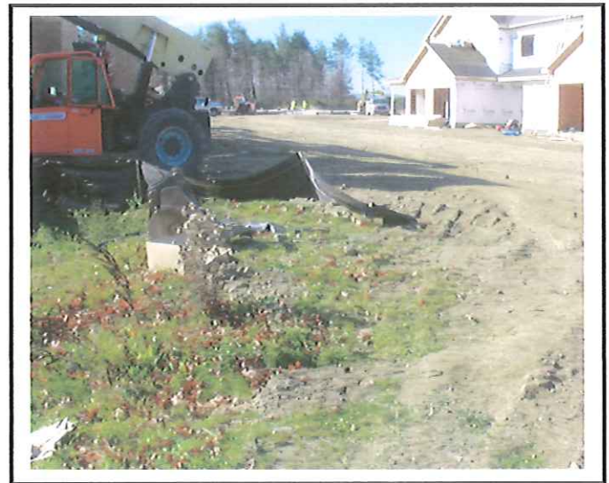
Additional silt fence is required around the stormwater practices.
