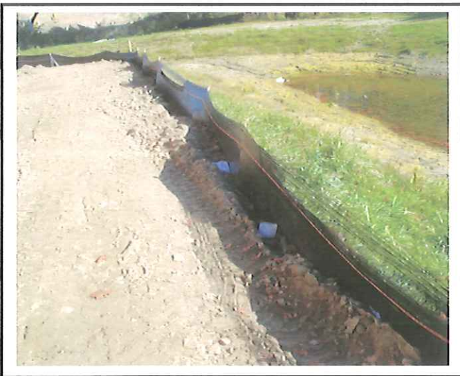
Silt fence is shredded and requires replacement.
