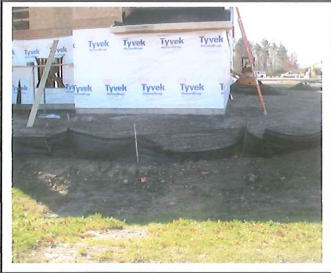
Silt fence is shredded and needs to be replaced.
