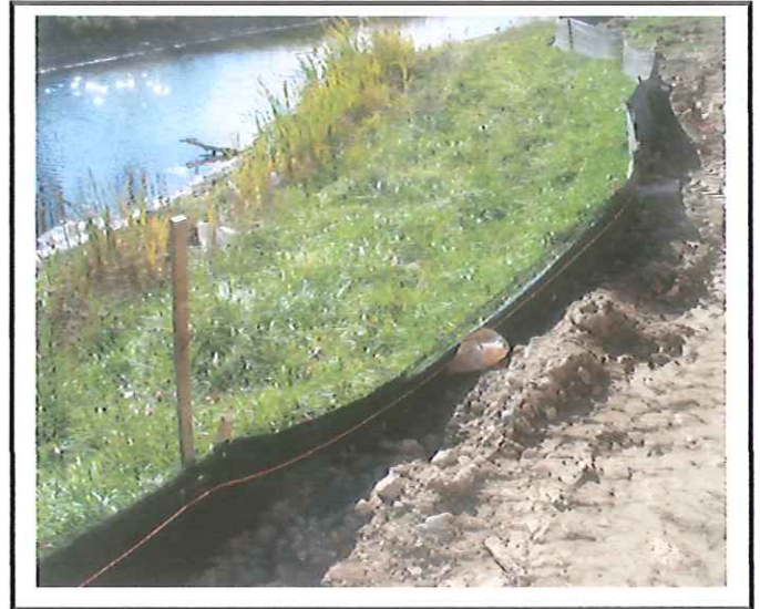
Silt fence is not installed according to standard and needs repair.
