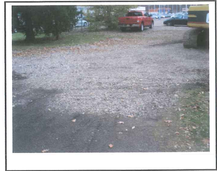
Construction entrance onto Fisherville Rd.- Equipment is blocking entrance so traffic is driving around it and off the construction entrance.
